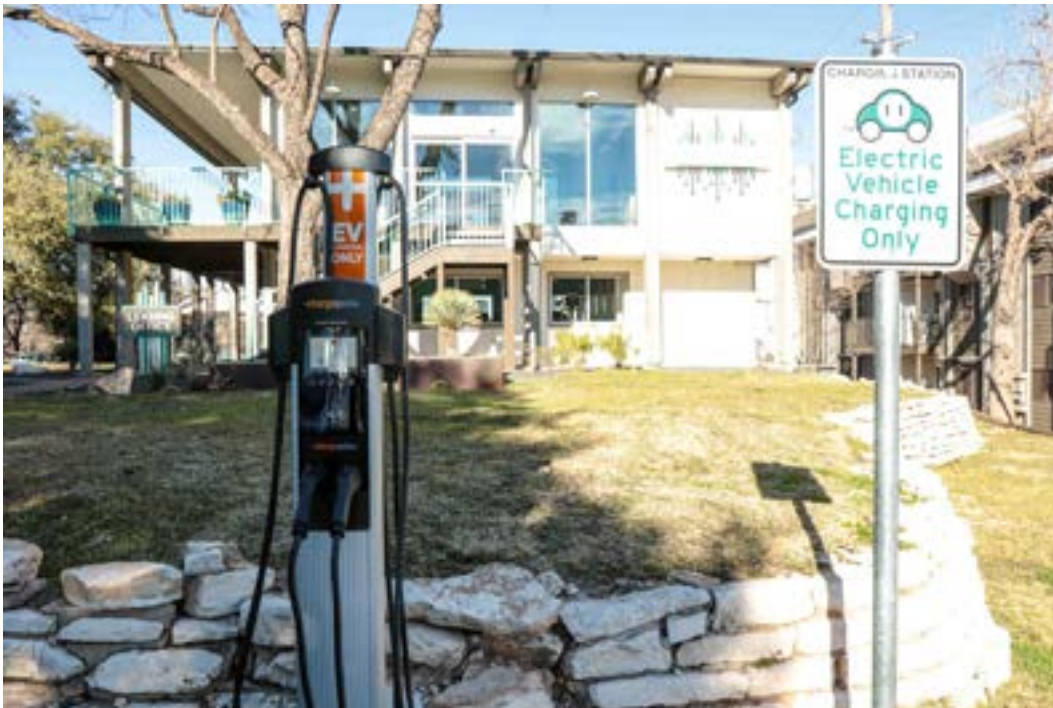
An Austin Energy charging station. Photo: Austin Energy ( https://austinenergy.com/ae/green-power/plug-in-austin/multifamily-properties/ )
