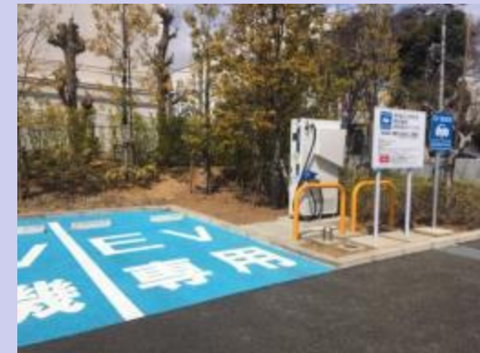
Fast chargers (Tachikawa Regional Office Building)
